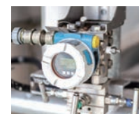
Water and gas meters
