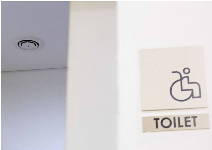
air-e nanoe™ X generator in a toilet in Paradigm Mall PJ.
