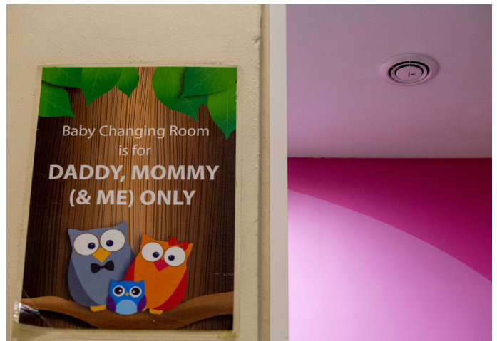
air-e nanoe™ X generator installed in a baby changing room in Paradigm Mall PJ.
