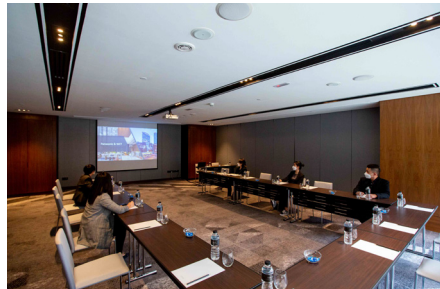
air-e nanoe™ X generator installed in a meeting room located at New World Hotel Petaling Jaya.
