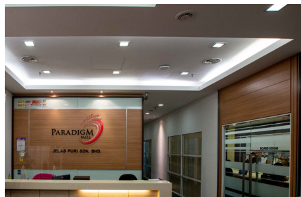
Installation of air-e nanoe™ X generator in the reception area located at Paradigm Mall management office.
