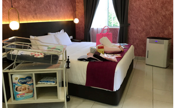
Installation of ziaino™ Air Treatment Unit in the bedroom.
