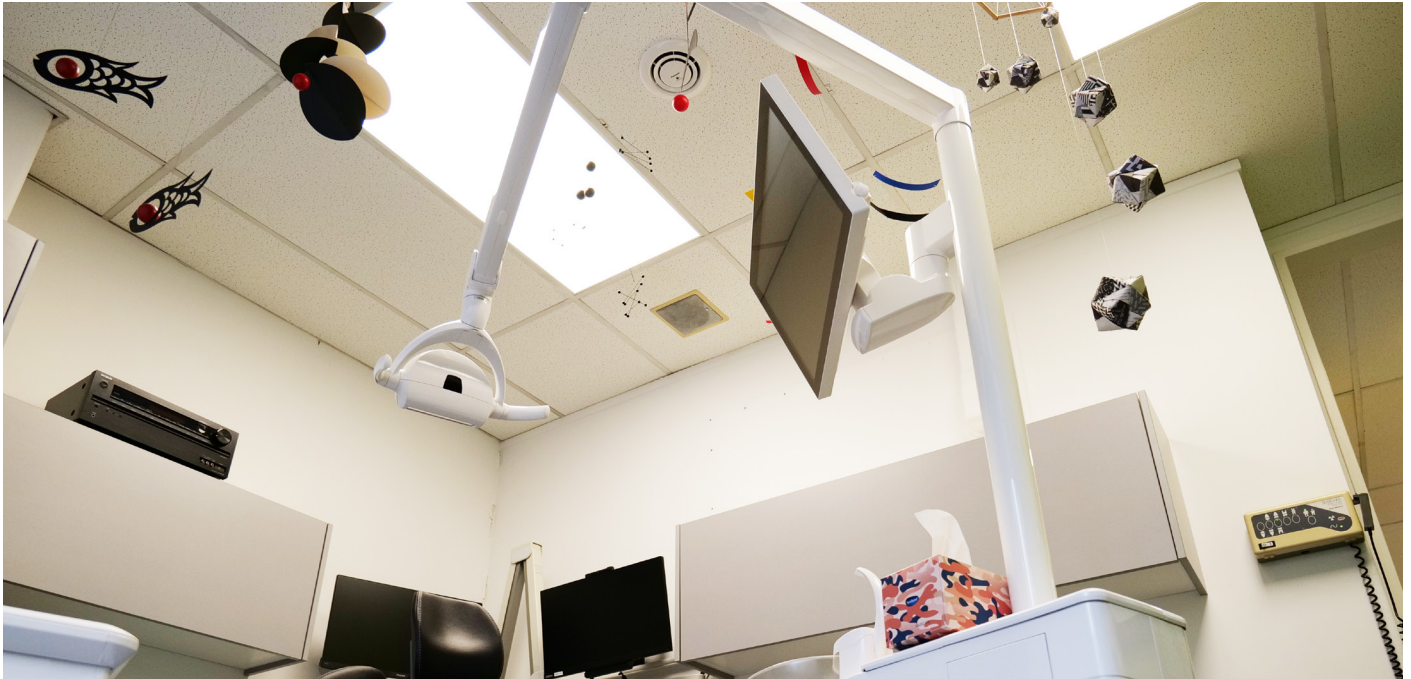
air-e ceiling mounted nanoe™ X generator installed in Queen Street Dental's treatment room.
