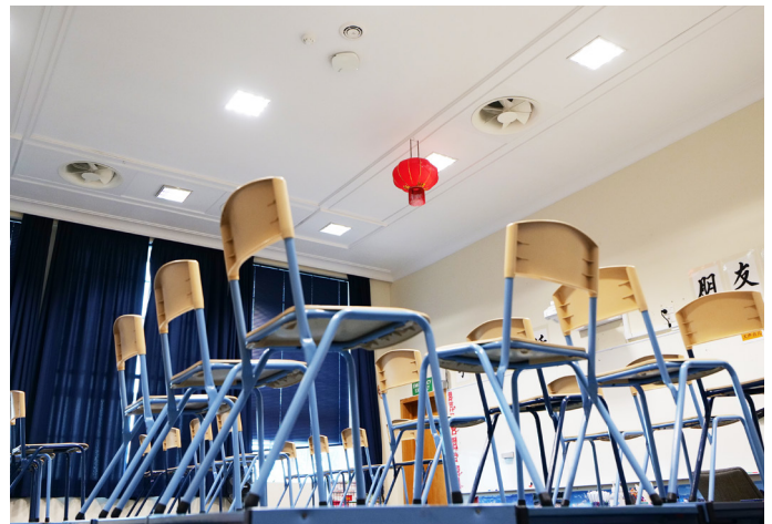
Neat installation of air-e ceiling mounted nanoe™ X generator.
