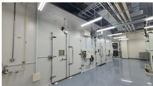
【simultaneous hot water and air conditioning multi-test laboratory】
