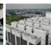
Outdoor units on the roof
