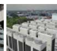
Outdoor units on the roof
